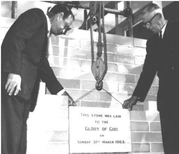
W R Bennett and F Edwards laying of foundation Stone for new hall 1963
